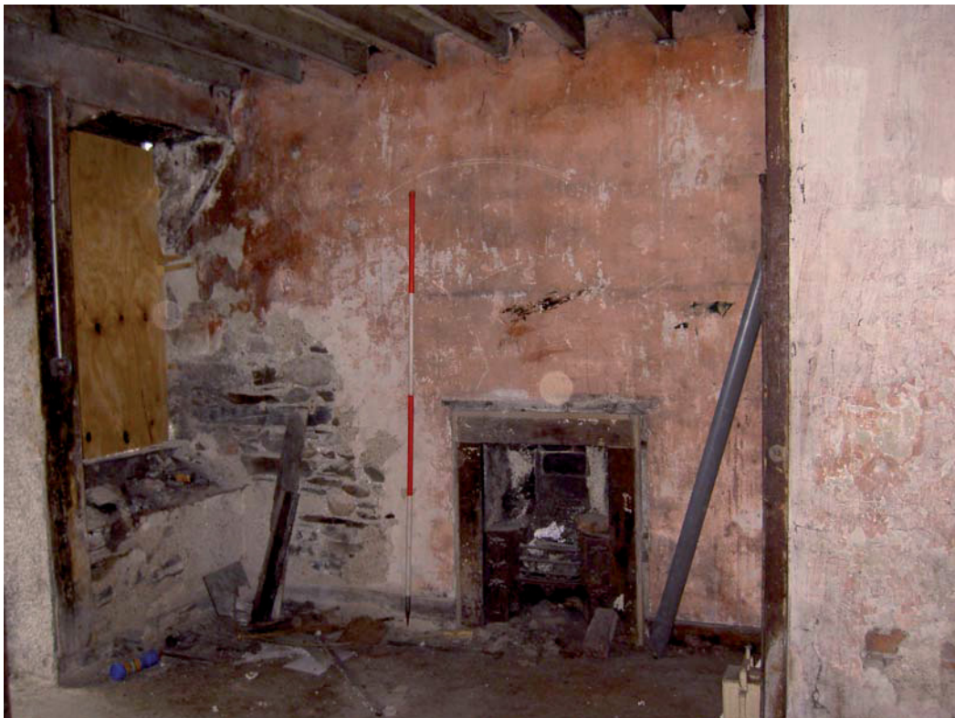
Plate 10: Ground floor east side, showing window, fireplace, and partition wall in north-east corner
