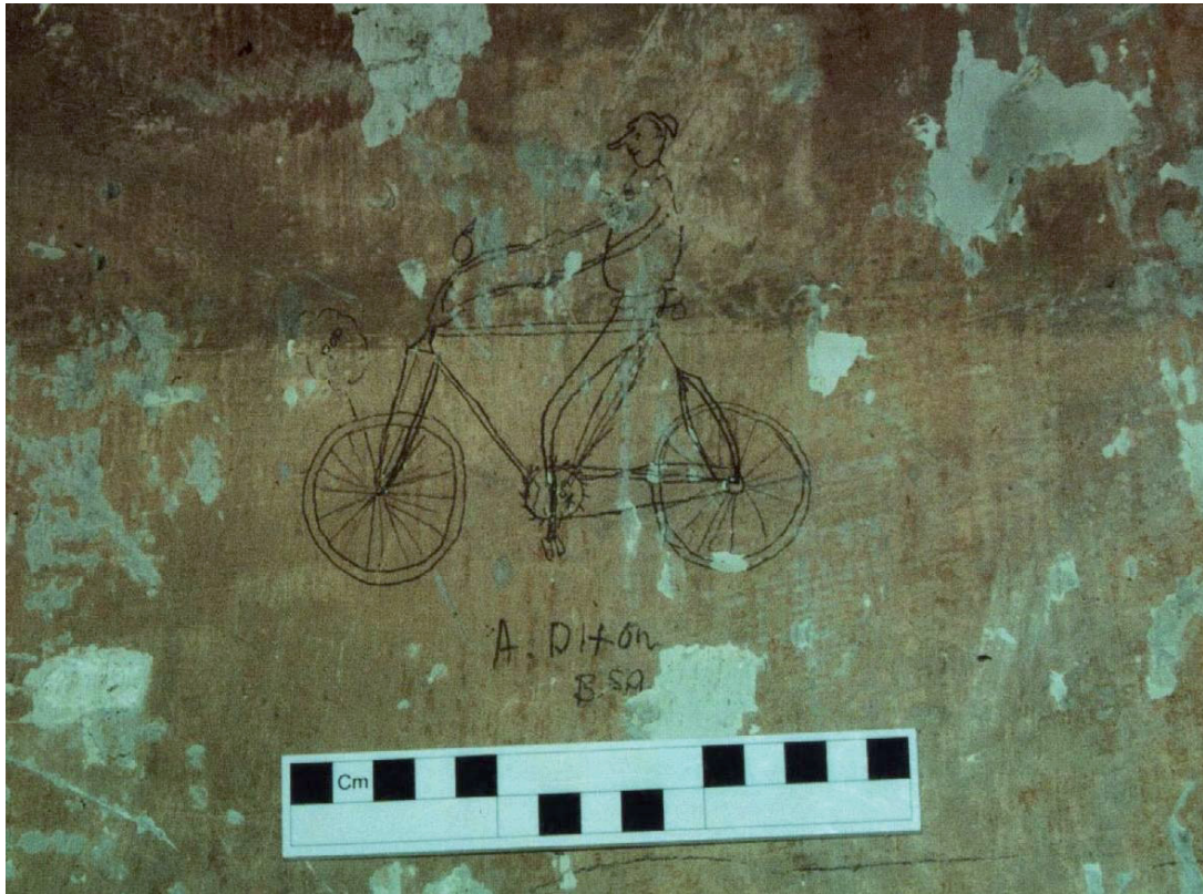
Plate 13: Graffiti by A. Dixon, puncturing a tyre on his BSA bike, on east wall of first floor
