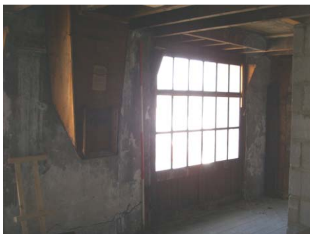
Plate 42: An 18-light window above vertical wooden slats fills the loading doors in the north elevation
