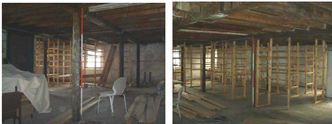
Plate 33: (left) General view of the north-east corner of the third floor showing the modern shelving and columns
