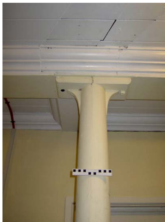
Plate 59: (right) Angled scar of the original wall visible in the ceiling ( Room 3 )
