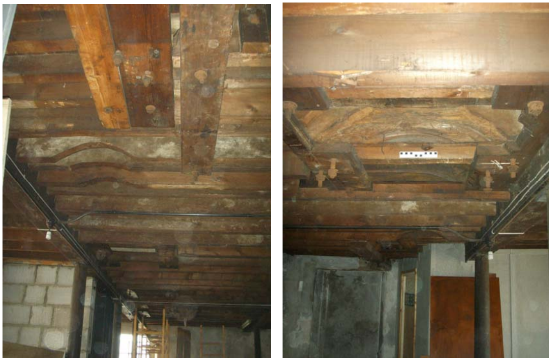
Plate 36: (left) The front (north) row of attachments and scarring to accommodate a drive shaft, showing where the joists have been purposefully cut
