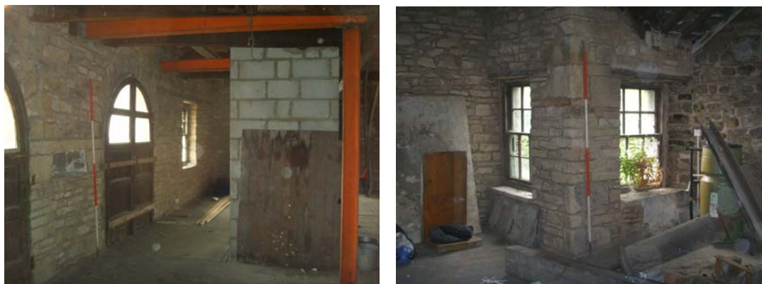
Plate 30: (left) Detail of the loading door and alcove in the north elevation
