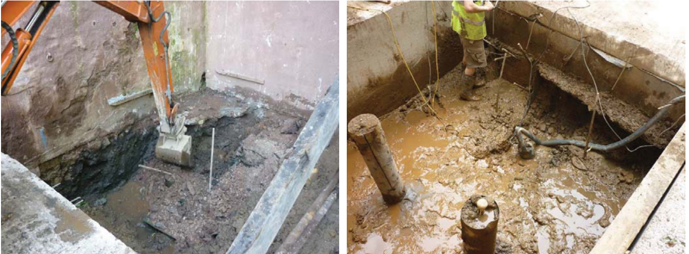
Plate 20 (left): Removal of the remaining floor in the south-east corner of the site
