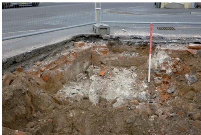
Plate 11: Concrete stanchion within the foundations of the building at the corner of Edward Street
