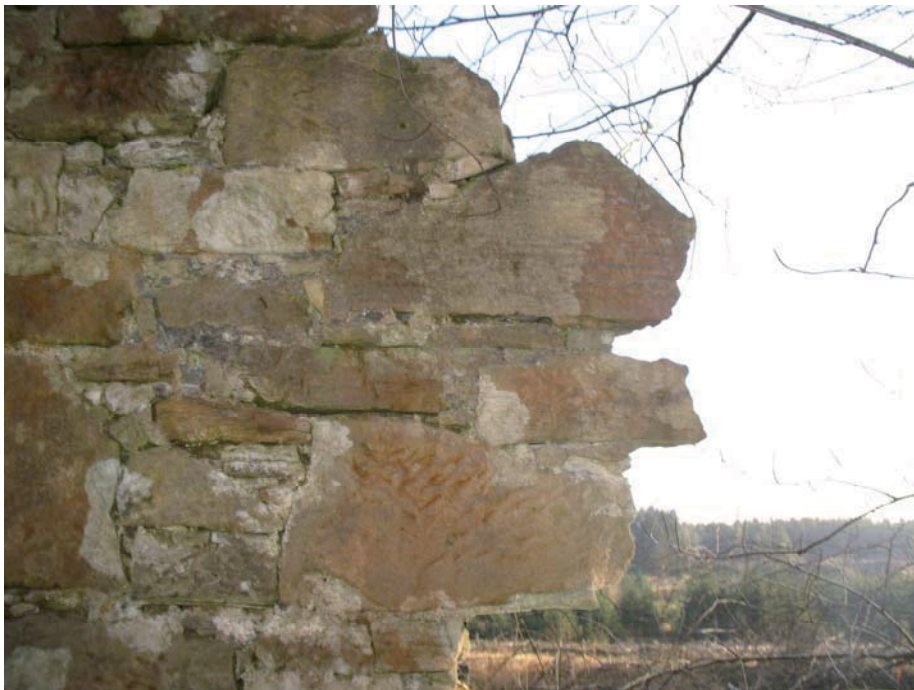
Fig. 15b: Detail of Skewputt, W Side of N-Facing Elevation, 201
