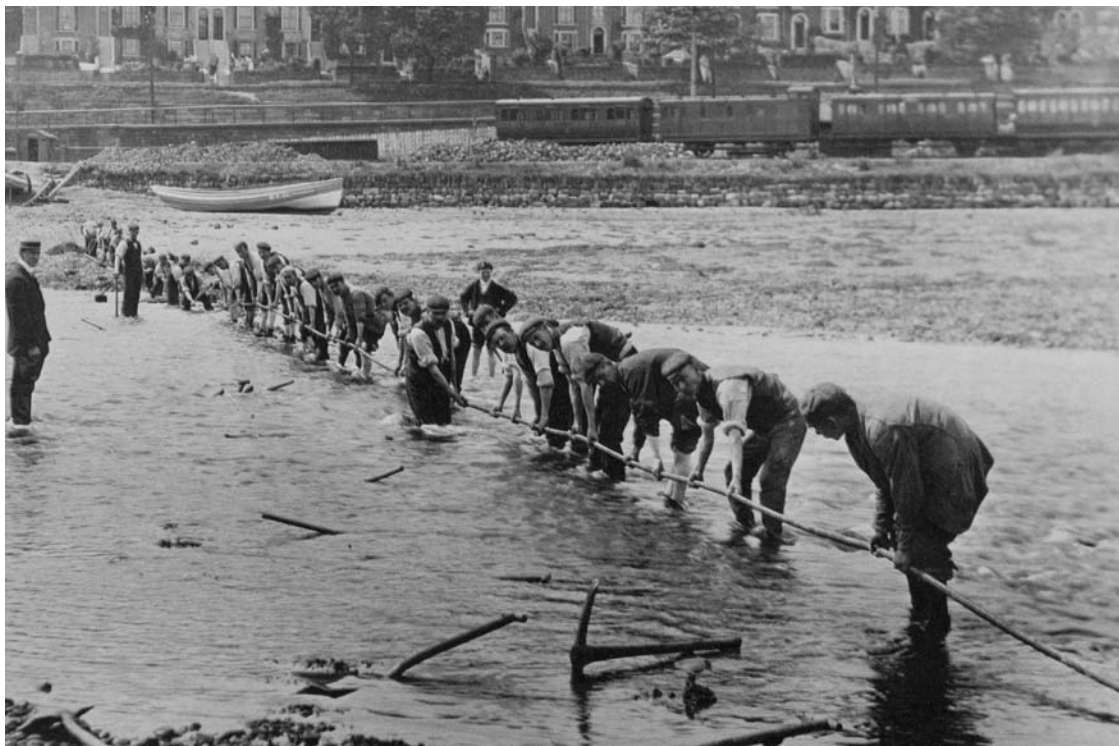
Figure 9.65. The laying of a cable in the River Esk (© Sutcliffe Gallery ( www.sutcliffe-gallery.co.uk ))
