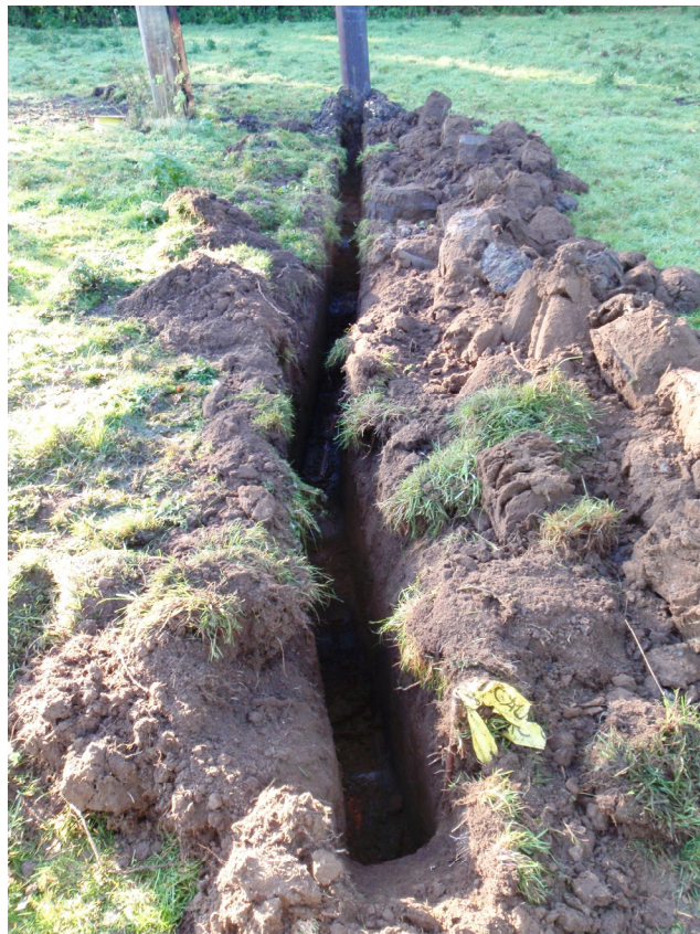
Plate 2: Trench extending to the north of new telegraph pole – with ceramic field drain to base
