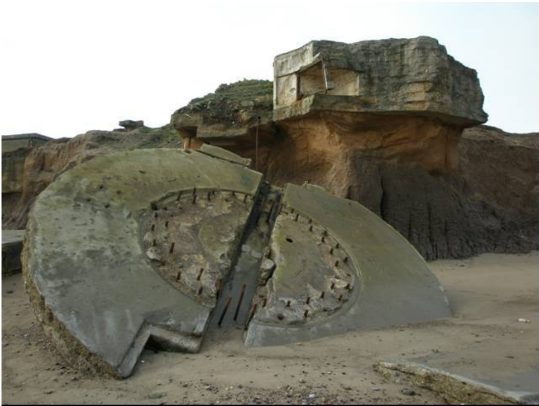
Plate 25 Collapsed 9.2in gun platform and precariously-balanced formerly-adjoining building, Godwin Battery, Easington (EA182), looking west
