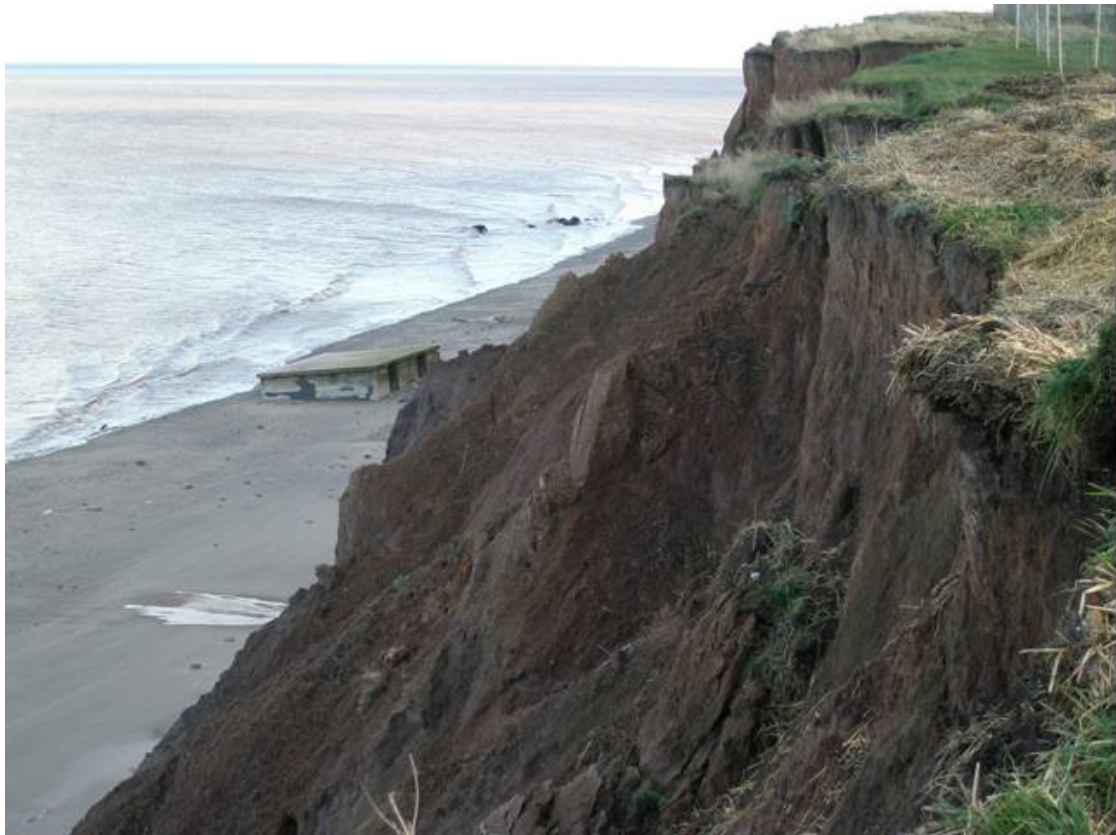
Plate 20 Eroding cliff edge, Aldbrough
