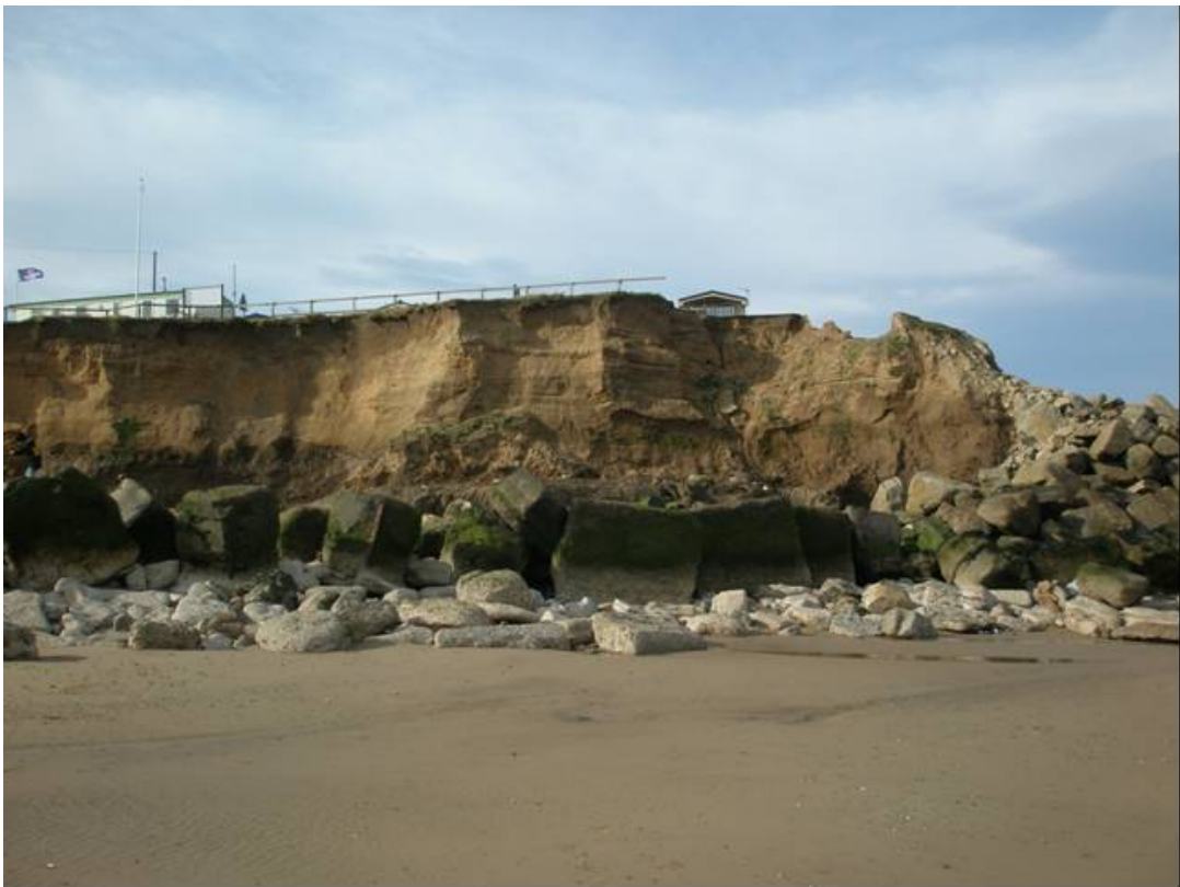
Plate 14 Local attempt at cliff protection using anti-tank blocks and rubble, Barmston
