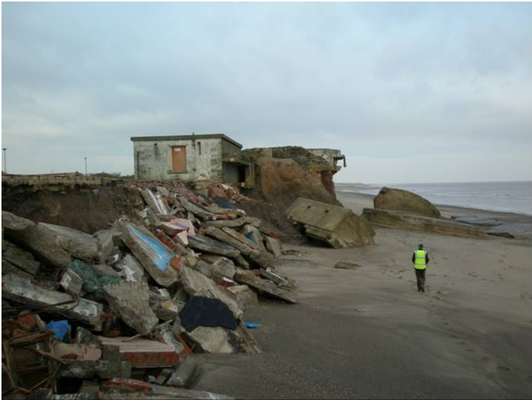
Plate 26 Line of recently-demolished shelters and workshops between 9.2in gun platforms, Godwin Battery, Easington (EA182), looking north
