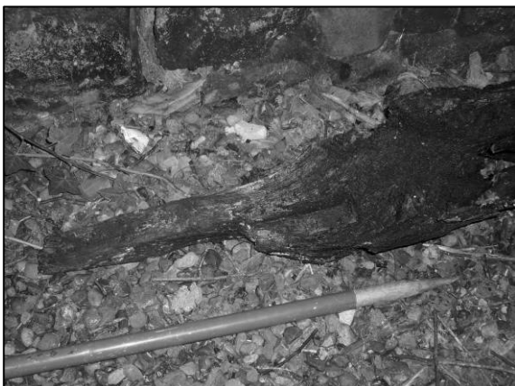
Photo 2/461: Timber 3 - detail of splayed scarf.
