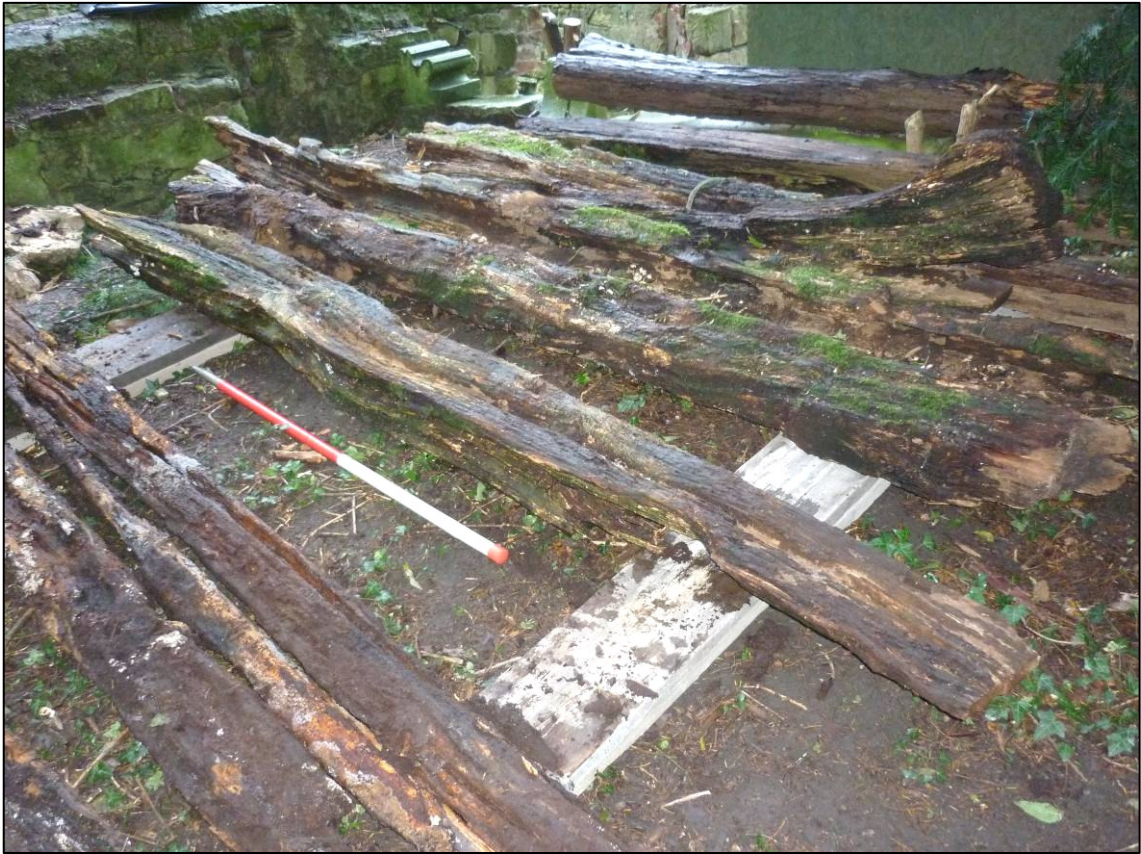
Plate 11: General view of old timbers after removal from west cell of gatehouse.
