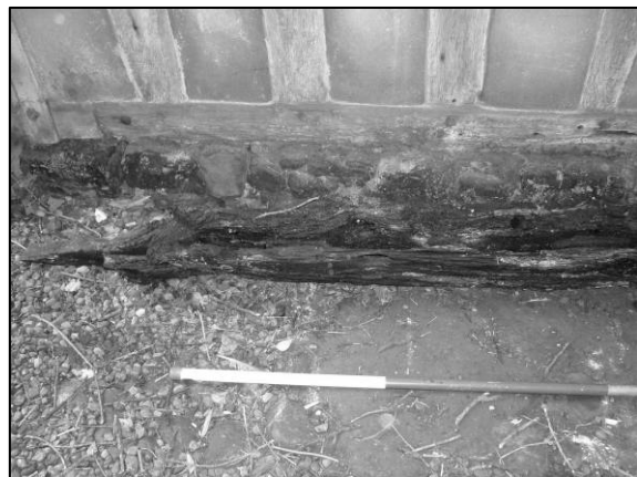
Photo 2/460: Timber 3 - detail of splayed scarf.
