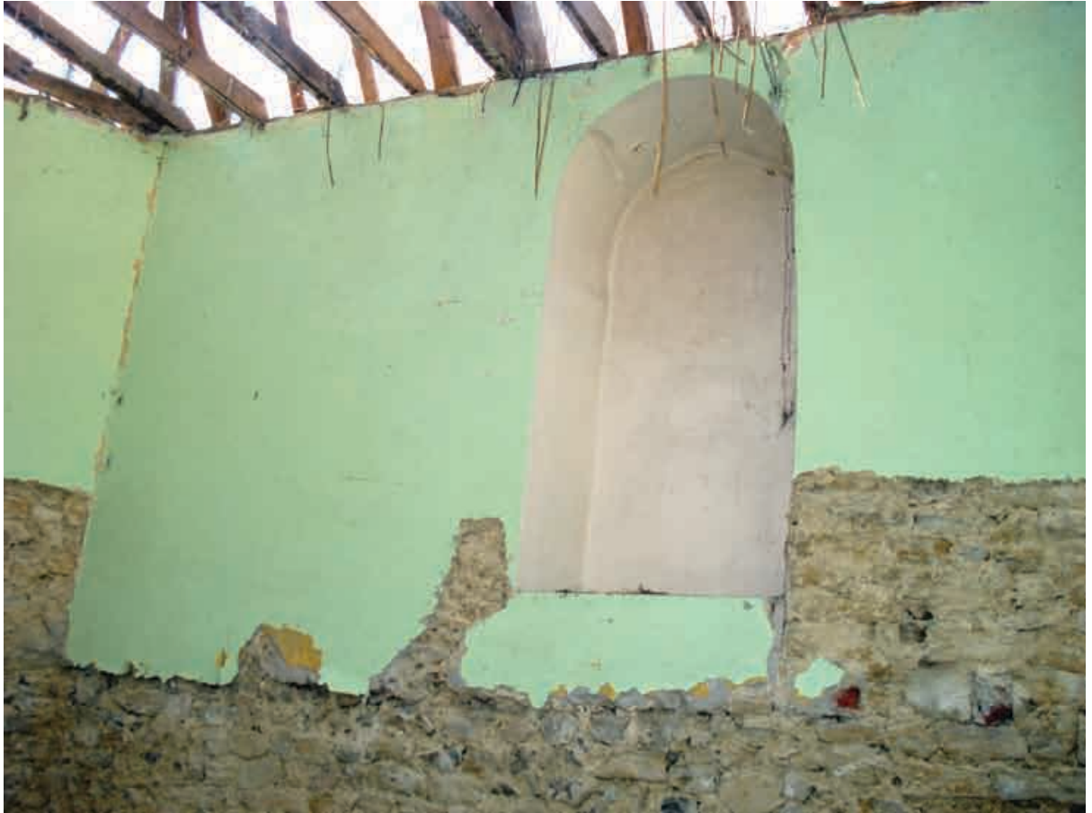
Plate 5 The blocked gallery doorway, showing infilling at bottom and floor-joist sockets blocked with bricks to right, looking northwest.
