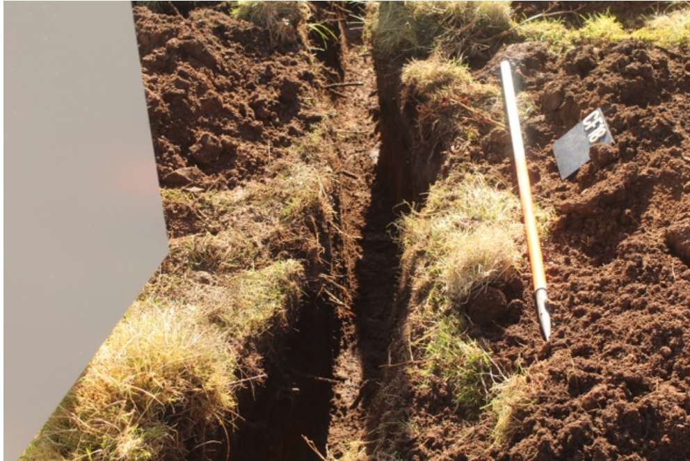
Illustration 5 Milquhanzie Hill, Crieff, Trench Spur from Electrical Box
