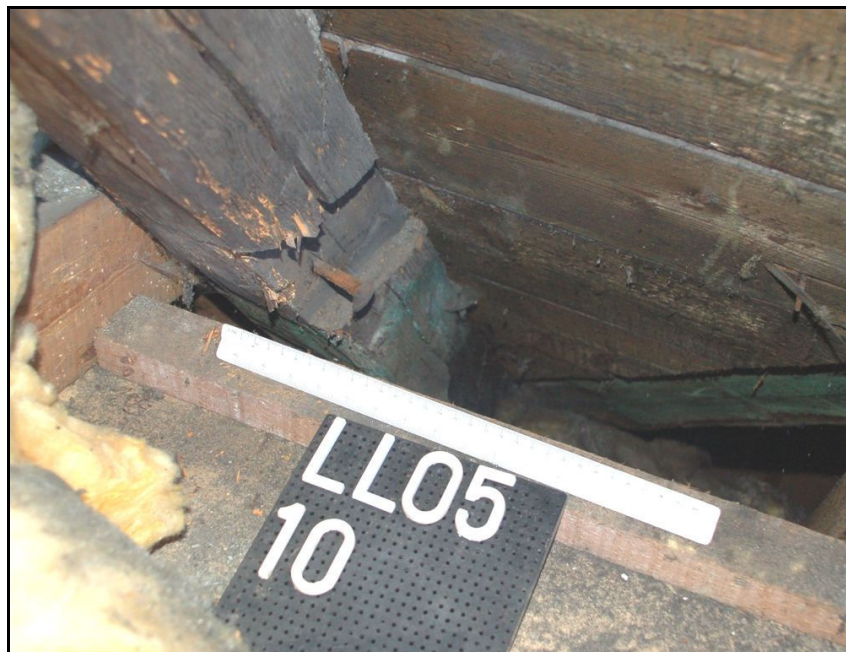
Photo showing lap joint where collar removed (rafter group 10) and iron spike/nail
