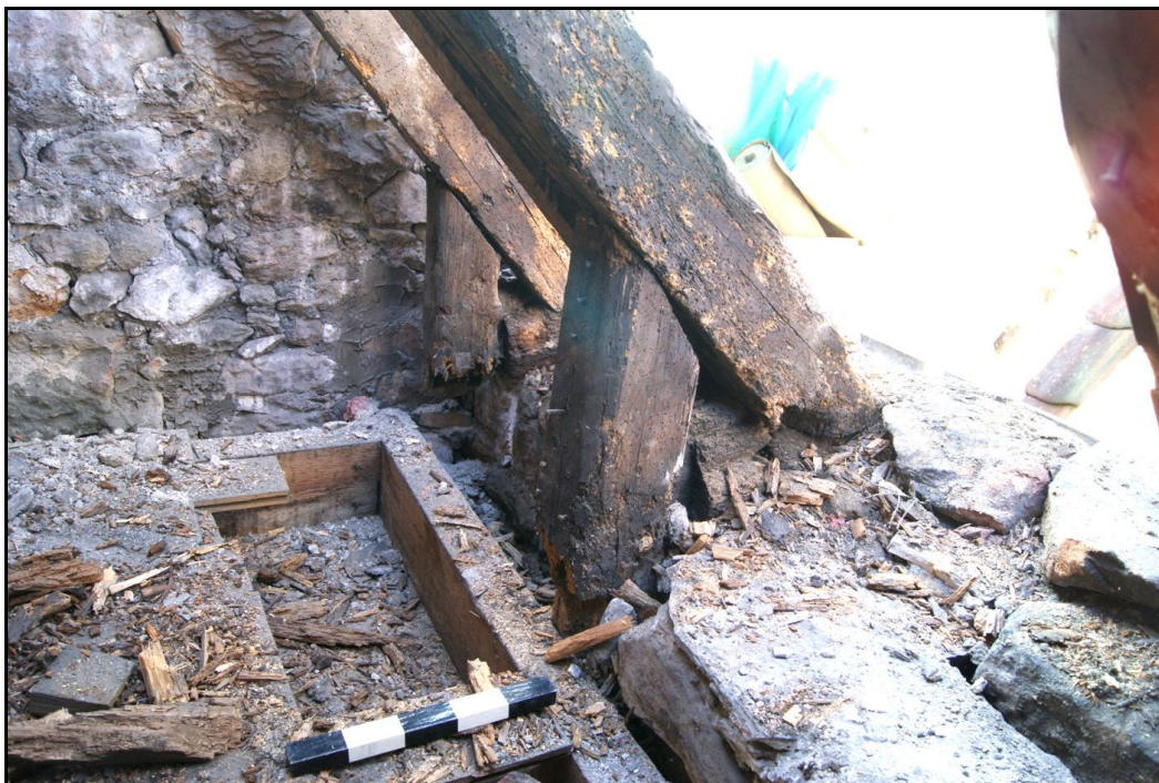
Photo showing ashlar posts on the W side of the S roof
