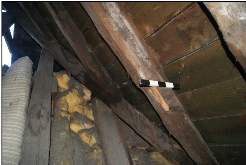
Photo showing a sawn off collar stub in the S roof
