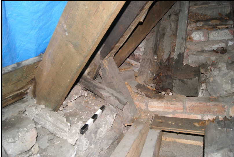
Photo showing that the ashlar post connected to rafter 17A as been pushed sideways due to the S roof spreading outwards
