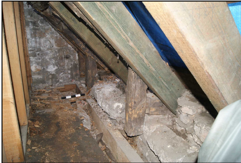
Photo showing replacement rafters on the W side of the S roof
