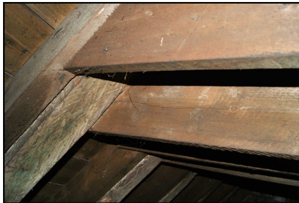
The double sets of modern collars nailed to the rafters in the S roof
