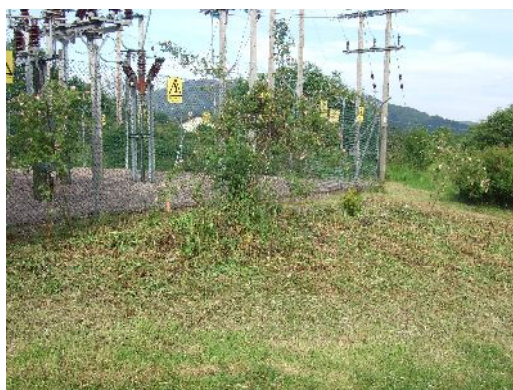
Rough ground around switching station (FW02_09)
