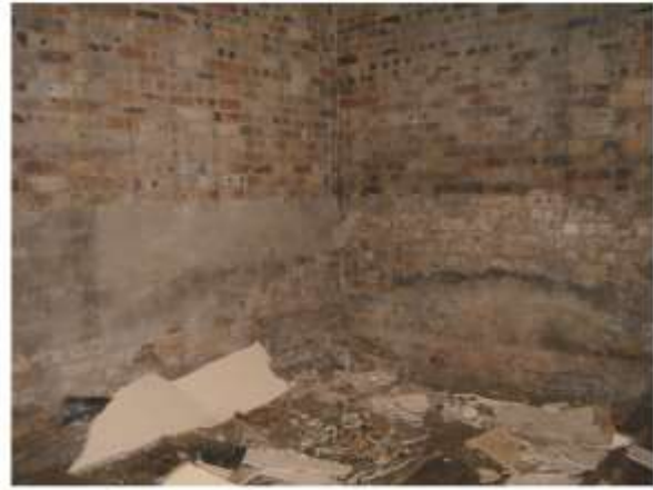
Image 023 NW corner. Cement scar on wall shows height of wall lining boards.
