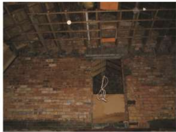
Image 029 North gable wall with doorway to balcony and balcony floor line on wall. Varnished roof timbers above ceiling beams.
