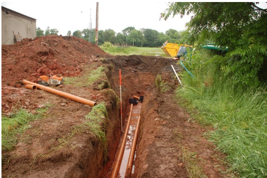
LF05_159 Drainage pipes into large deep excavation for inspection chambers, view NNW
