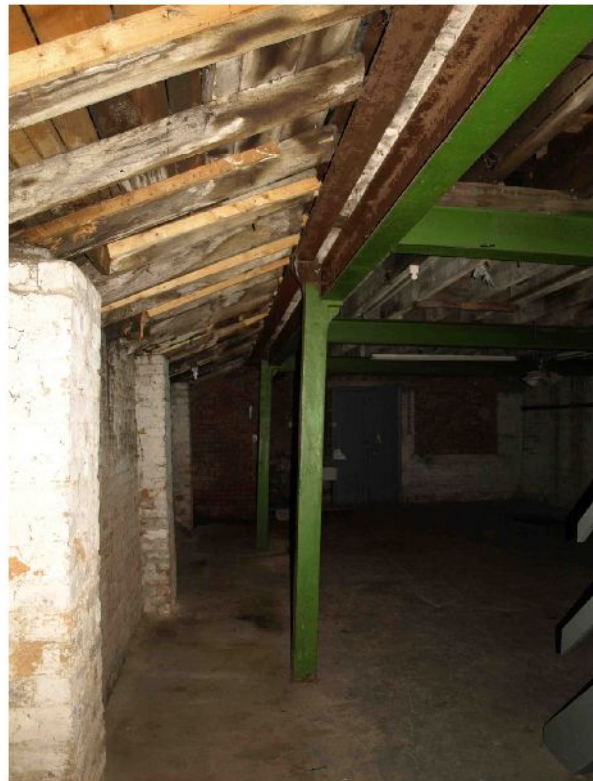
Illus 9 Banks interior. Green-painted cast-iron columns 011, rolled steel joists 010, replace W wall. Lean-to roof on W.
