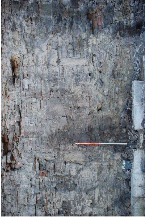
Illus 13 Watsons. W face of Wall 007. Blocked opening 032, with imprint of timber lintel above and iron bolt and washer 031.
