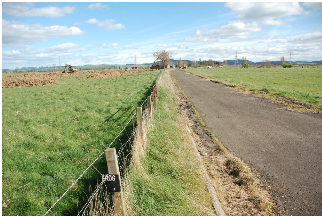
Illus 5: General excavation of trenches and disused road through site, view SE
