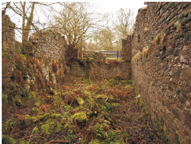
Illus 8 Mill House 02 interior. W Wall 03 ahead. Pit 23 and Wall 11 under vegetation in foreground. Wall 04 to R with Scarcement 10 and Putlogs 15 - 20 below.
