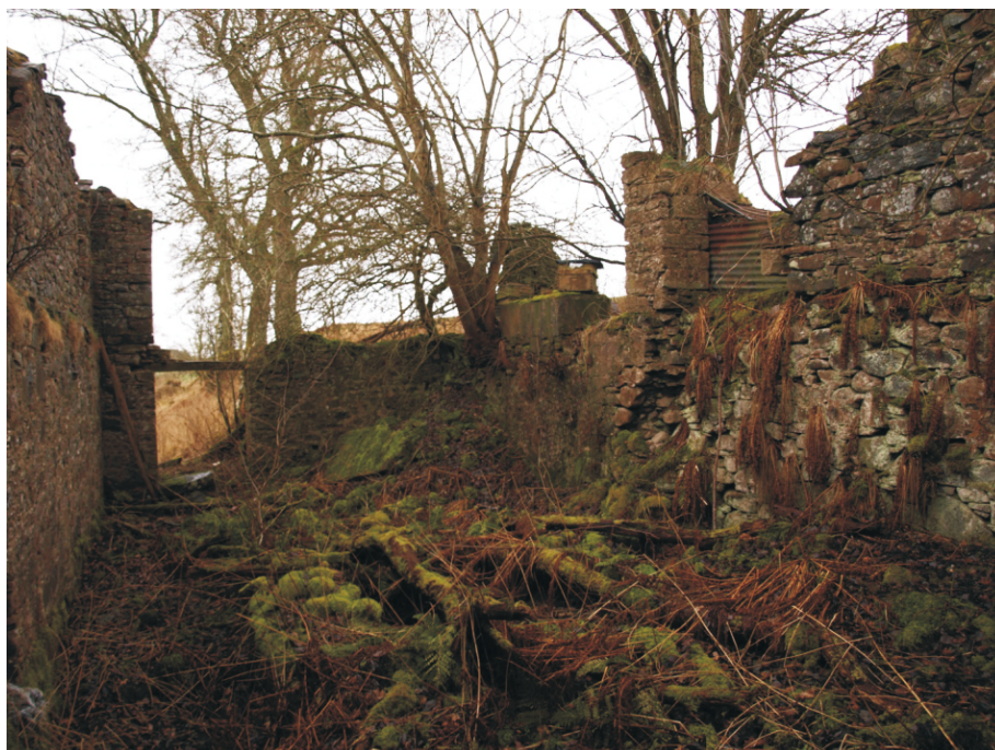
Illus 11 Mill House 02 interior. E Wall 05 and Lintel 22 ahead. Pit 23 and Wall 11 under vegetation to L. Concrete Plinth 30 on S Wall 06.
