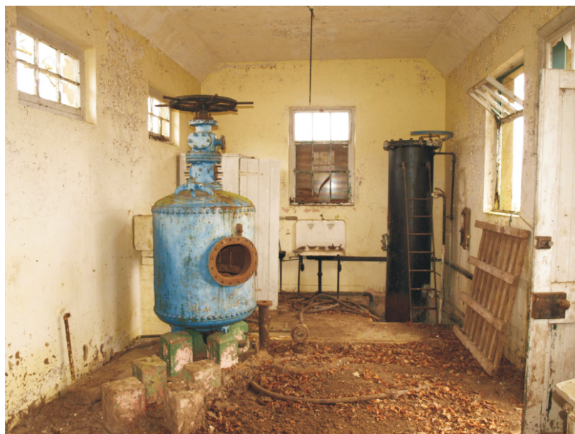
Illus 13 Water Treatment House 34 interior. Machine 38.
