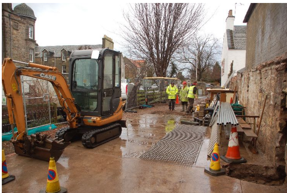
Illus 3: General of site showing concrete floor at N end, view N
