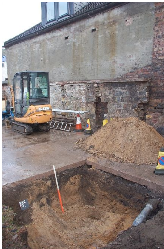
Illus 7: Evaluation pit 03 showing concrete floor and makeup over natural sand, view NE
