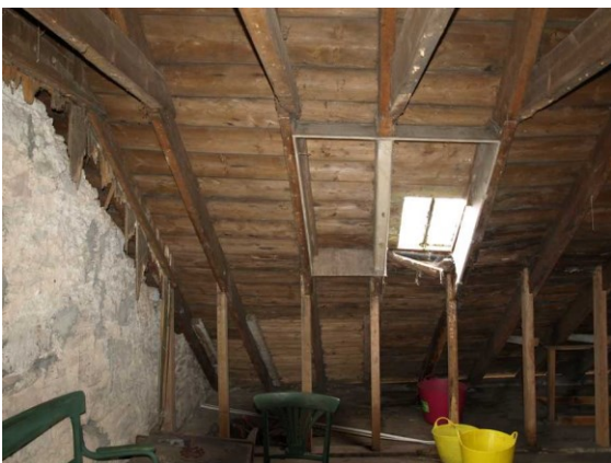
Illustration 17: Reduced roof light in NW corner. Traces of lining boards on W gable wall.
