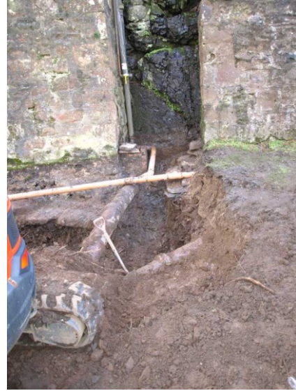
Illus 11 Foundation 014 and slab 020 under tower and buttress. Oily cliff face. Fuel filler pipe on side of tower.
