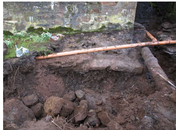
Illus 8 Foundation 014 and slab 020 under tower and buttress (R). Bedding 015 and rubble 012 under foundation 014.
