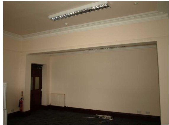
Illustration 15: Ground Floor, NW Room. Modern glazed entrance door. Long alcove in S wall. Deep beam overhead, reduced ceiling. Corniche and picture rail follow main high ceiling. Simpler cornice in alcove.
