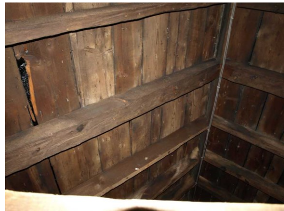
Illustration 25: Rafters and sarking boards. Double thickness rafter overhead, with interrupted ridge beam.
