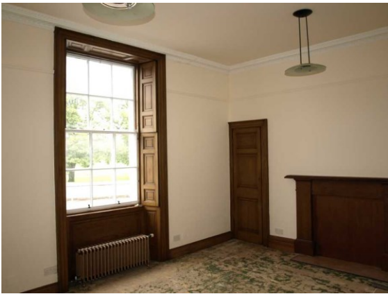
Illustration 12: Ground Floor, NE Room. Window shutters. Oak finish fire surround. Moulded plaster cornice.
