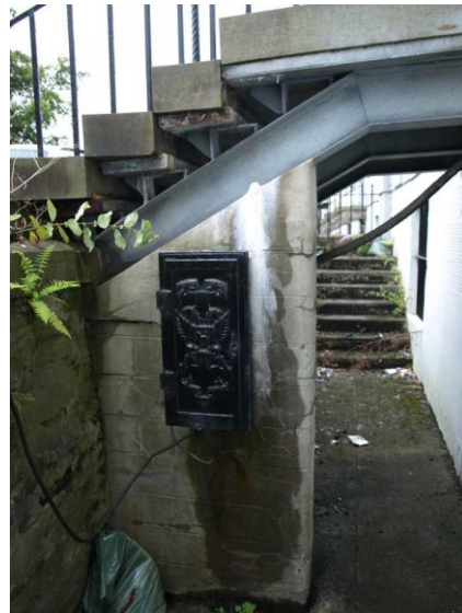
Illustration 30: Front Area. Steel sub-frame and cast iron switch box.
