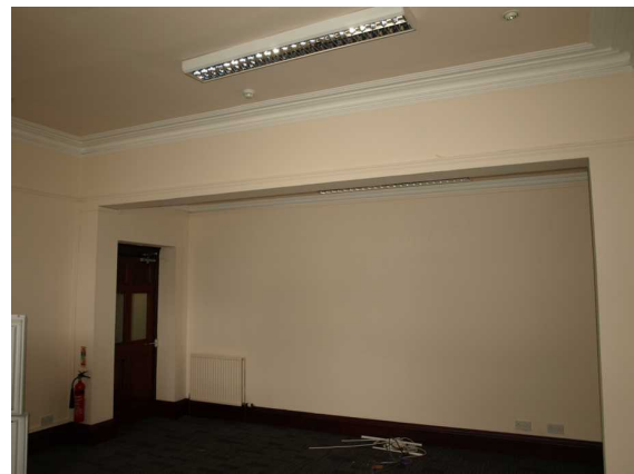
Illustration 15: Ground Floor, NW Room. Modern glazed entrance door. Long alcove in S wall. Deep beam overhead, reduced ceiling. Cornice and picture rail follow main high ceiling. Simpler cornice in alcove.
