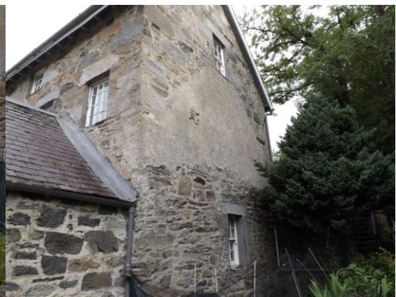
Possible roof ghost over wheel pit
