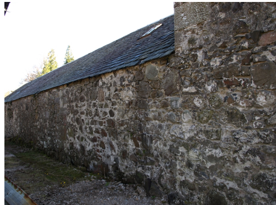
Illus 14 W elevation, S end. Changes of build. Junction of courtyard wall.
