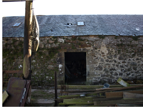
Illus 13 W Elevation. Store room door. Repointing, and change of build above lintel.
