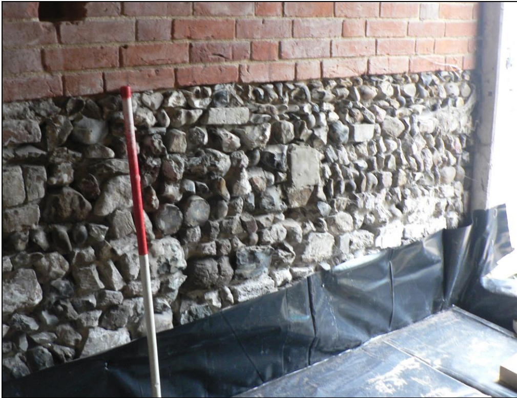
Post medieval flint wall on east side of eastern range containing Post medieval brick- probably part of garden wall earlier than 19 th century outbuildings
