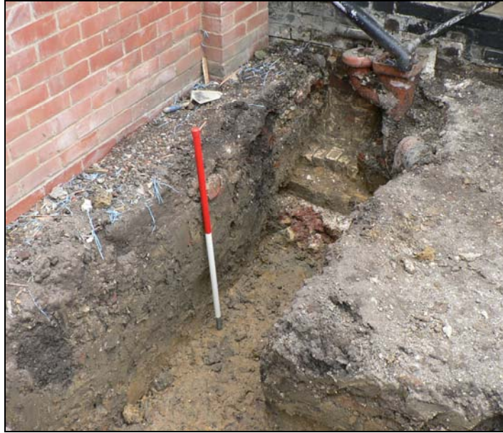
Eastern footing trench from north-west showing ditch 0002 in long section & deep existing house footing over the line of the feature below the pipes
