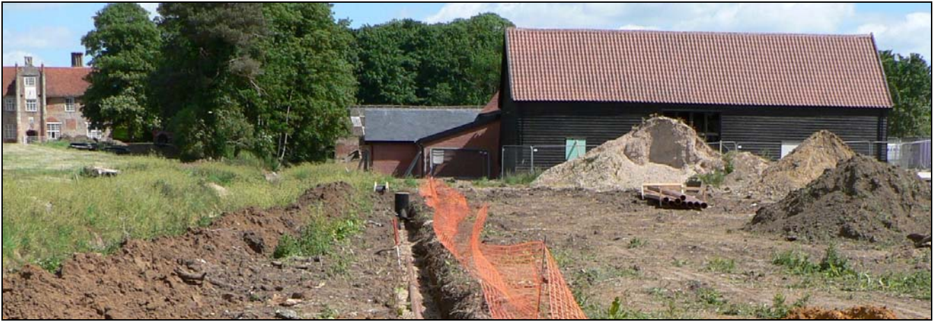
Image 1- site from south with Bruisyard Hall to left and farm complex to right
