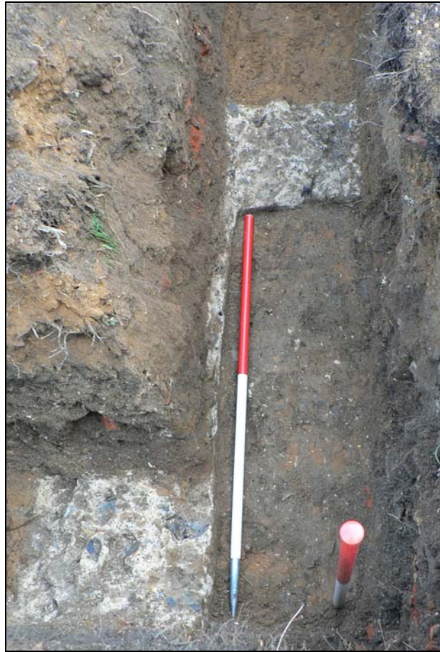
Walls 0004 & 0005 in side extension footing trench from north-west (as left in situ)
