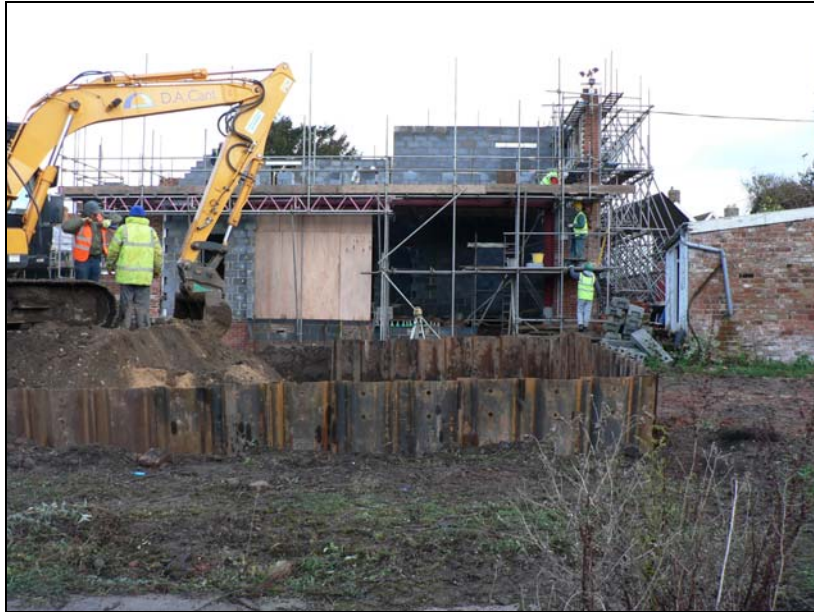
Site from west with steel sheets in place (and house being reconstructed in background)
