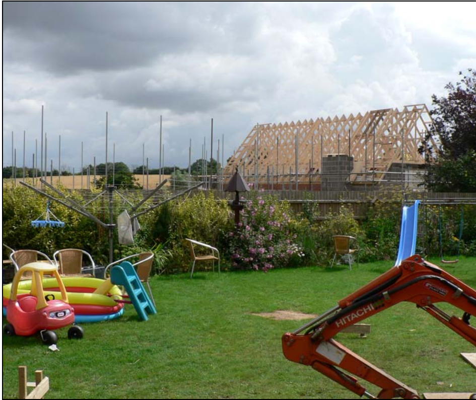
General view across back garden looking east- note garden level in relation to roof line of new build on area of DBN 132
