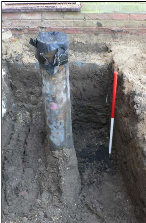
Excavation of ground beam trenches from west- showing top of peaty deposit at base
