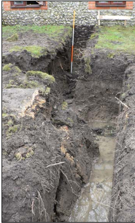
Foundation trench close to stables building with collapse
