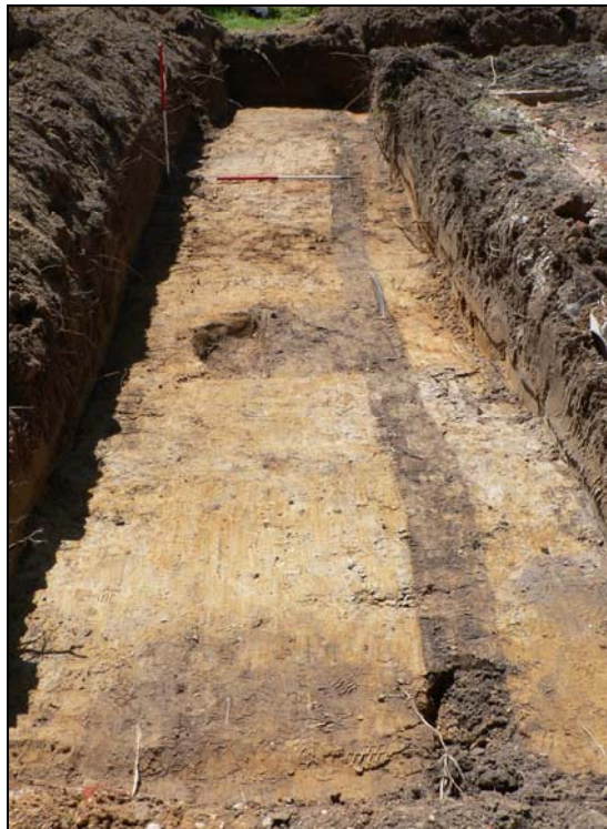
Trench 1 from north with pipe trench & tree root pit at mid point
