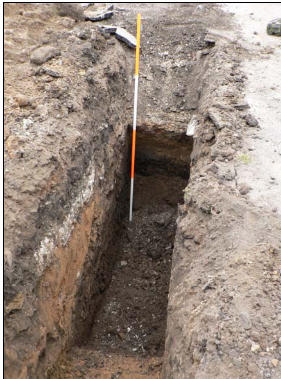
Internal foundation trench from south dropping into late Pmed pitting & with chalk surface in left to section
