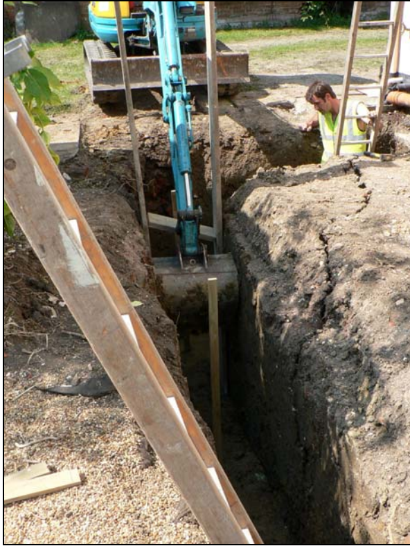
North-western corner of foundations with crack showing edge of filled-in pond arm
