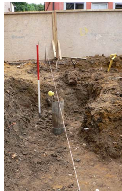
Area of pitting in north-west corner
