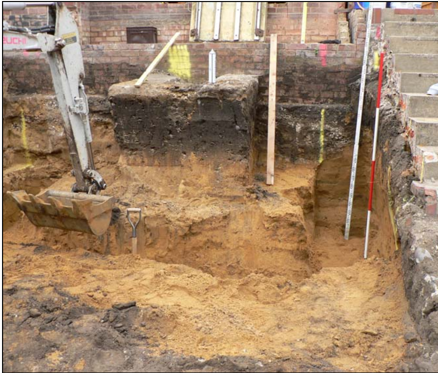
Removal of material deposited at the rear of the house during the original construction works
