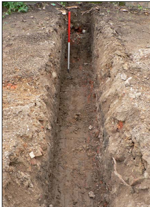
Eastern foundation trench for garage with later Pmed deposits in profile at end
