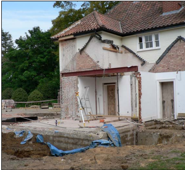
North-west corner of hall from SW showing late 20 th C cellar foundation
