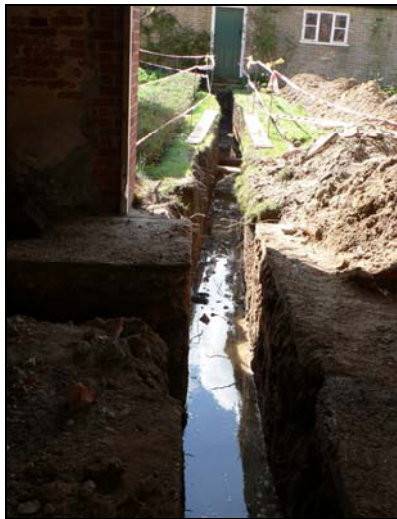
Pipe trench running across enclosed garden to the south of the Coach House
