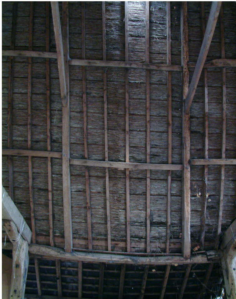
Photo 2.22 Butt-purlin roof with sagging rear wall-plate over the rear central bay
