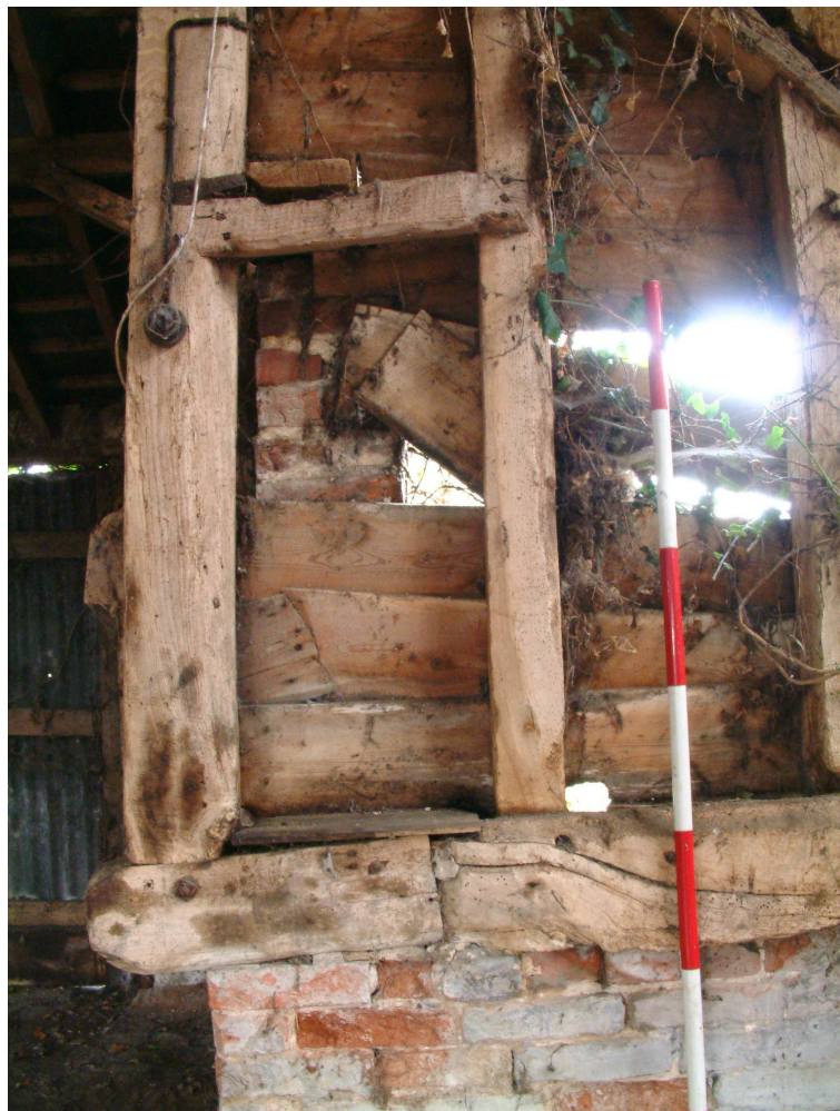
Photo 2.15 Altered primary timber post and rear sole-plate by the rear central bay
