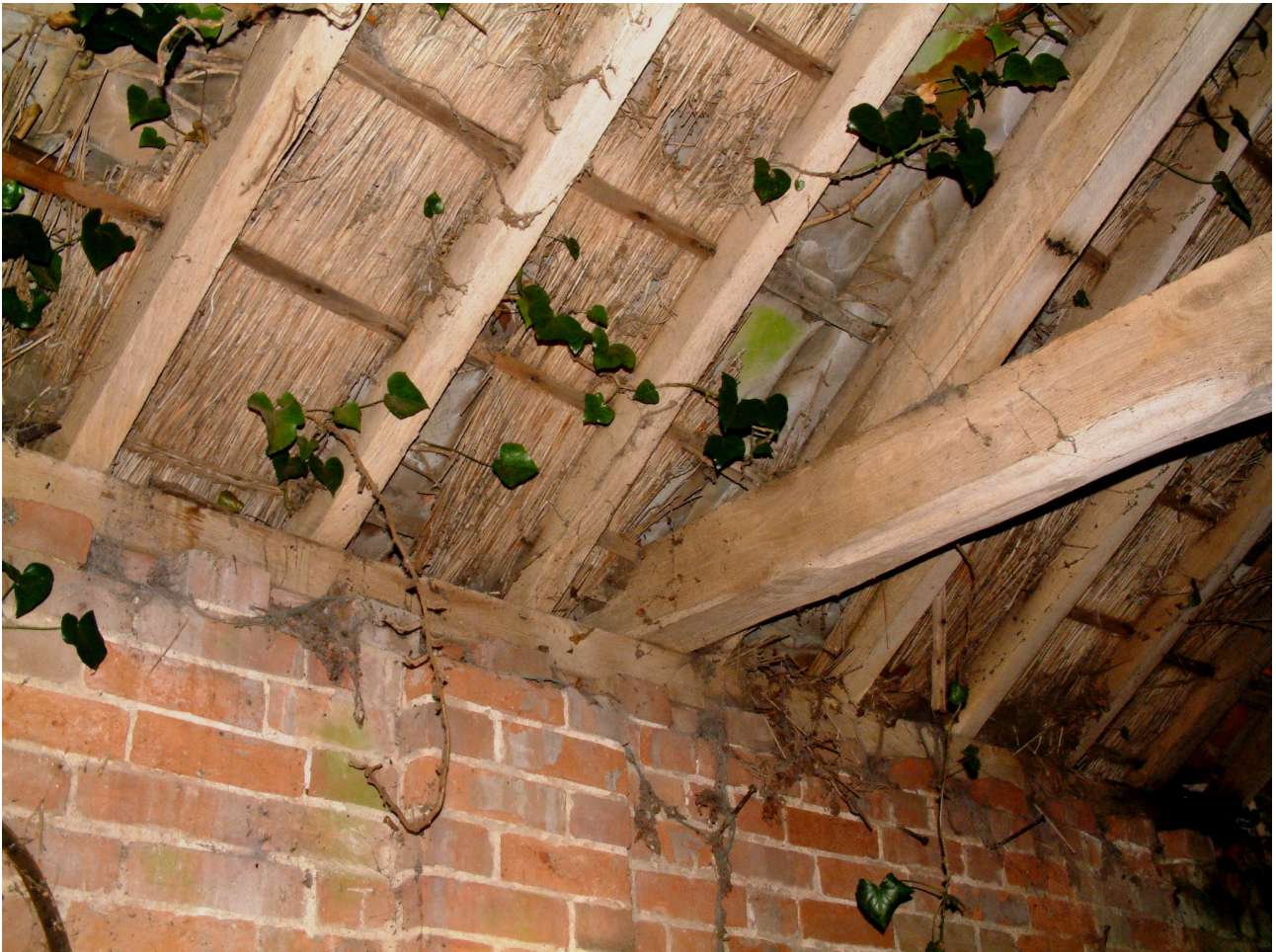
Photo 6.8 Inner face of brick eastern wall with pier, dentil decoration and roof
