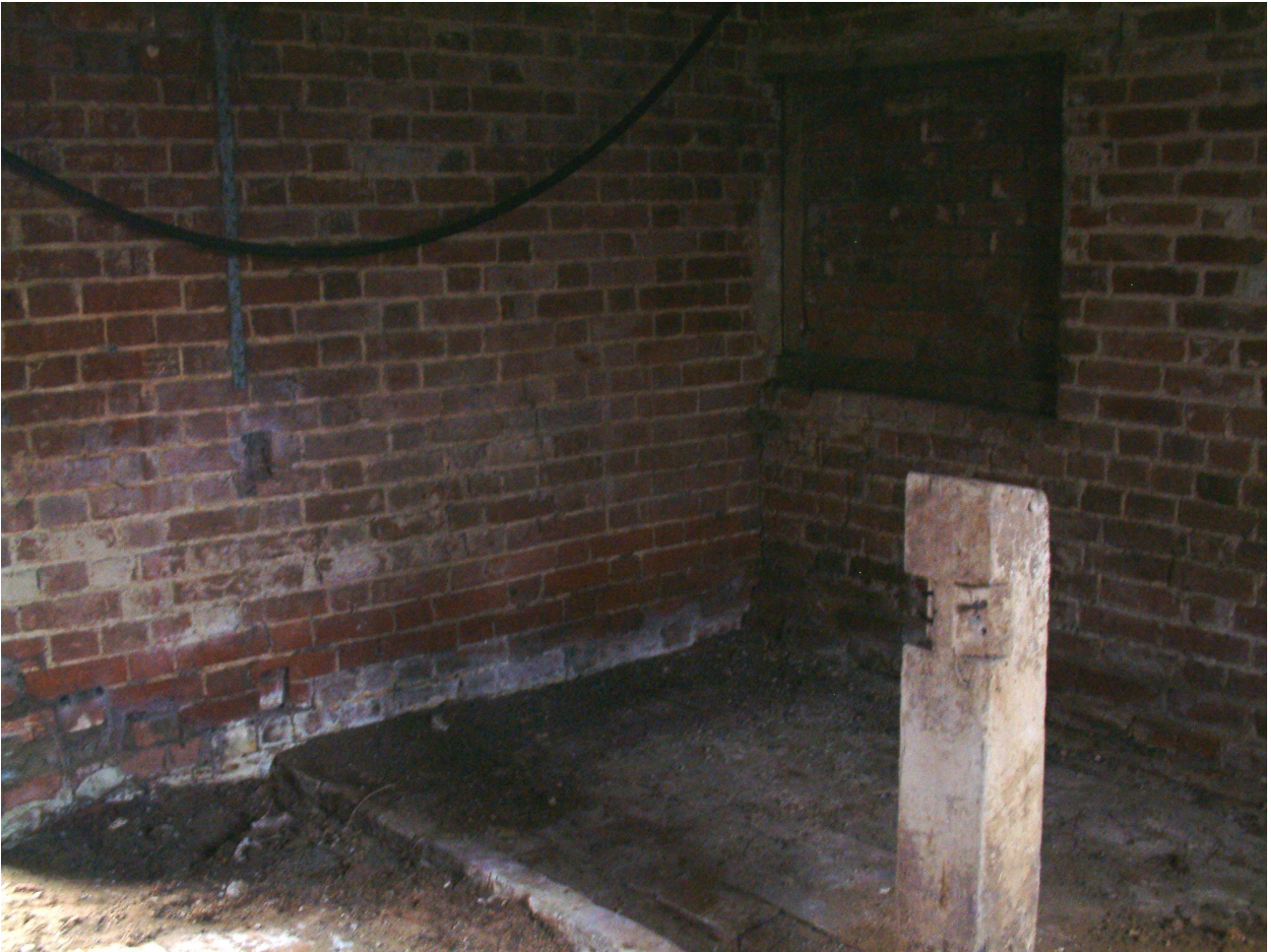
Photo 5.2 The remains of the fence with the blocked hatch in the west wall
