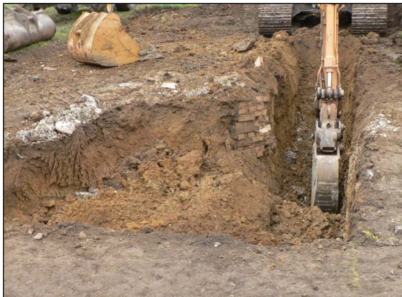
Ground works for new tank with 300mm topsoil over 450mm subsoil and 20 th century manhole brickwork exposed
