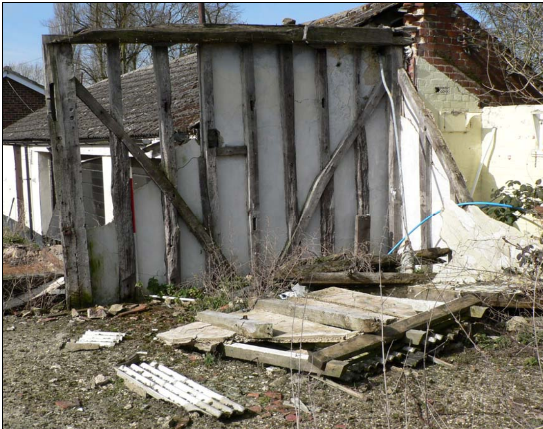
Remnant of timber framing surviving at eastern end of cart lodge to east of bungalow from south-east
