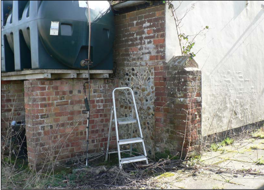
North-west corner of 19 th century cart lodge remnant to east of bungalow
