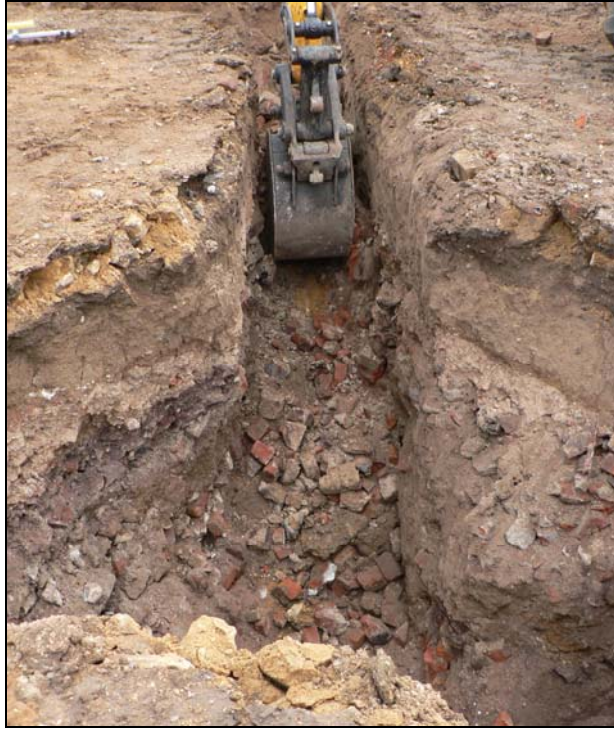
Foundation trench through brick built below ground oven base near centre of new house footprint from west
