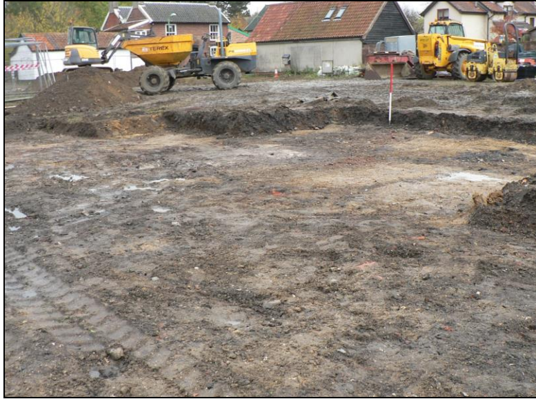
Maximum depth of soil strip in the central part of the site
