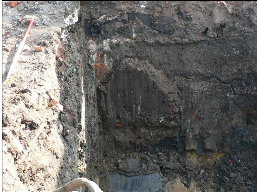
Deposit profile following removal of fuel tank in central part of the site
