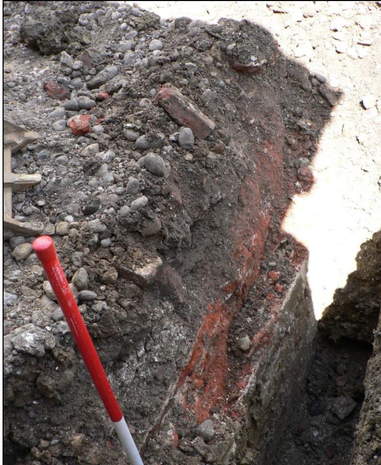
Initial trench excavation on eastern side of northern extension area with cellar wall partially exposed
